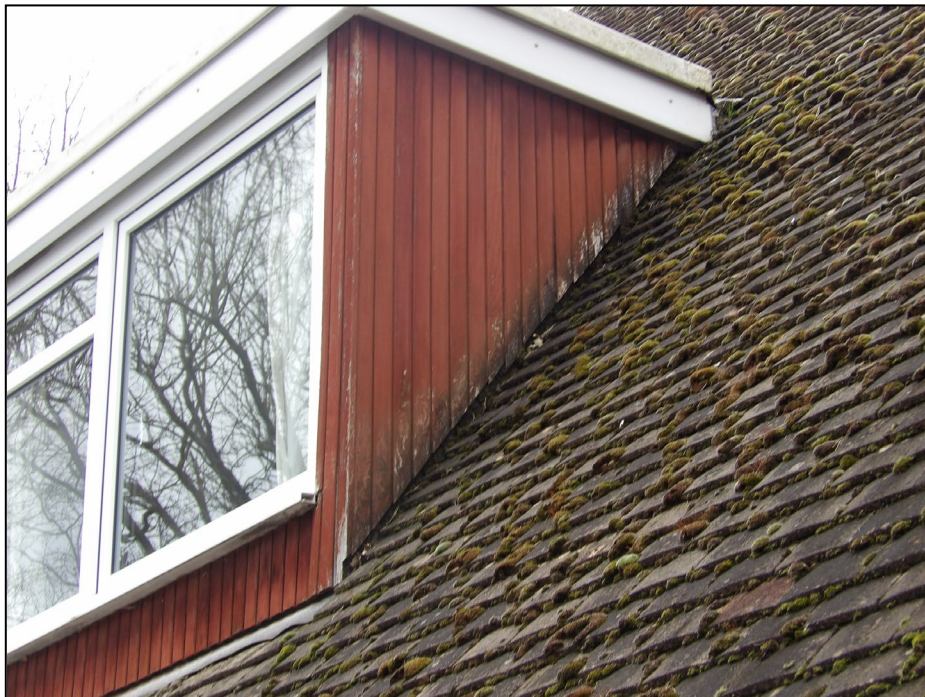
Figure 9. Close fitting wooden cladding and sealed fascias on dormer. 5 Greenside, Crowthorne. 17.03.26
