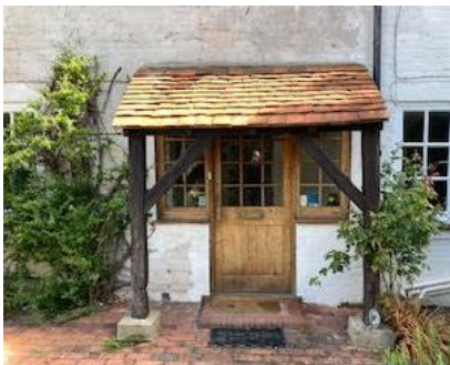
Existing poor quality porch
