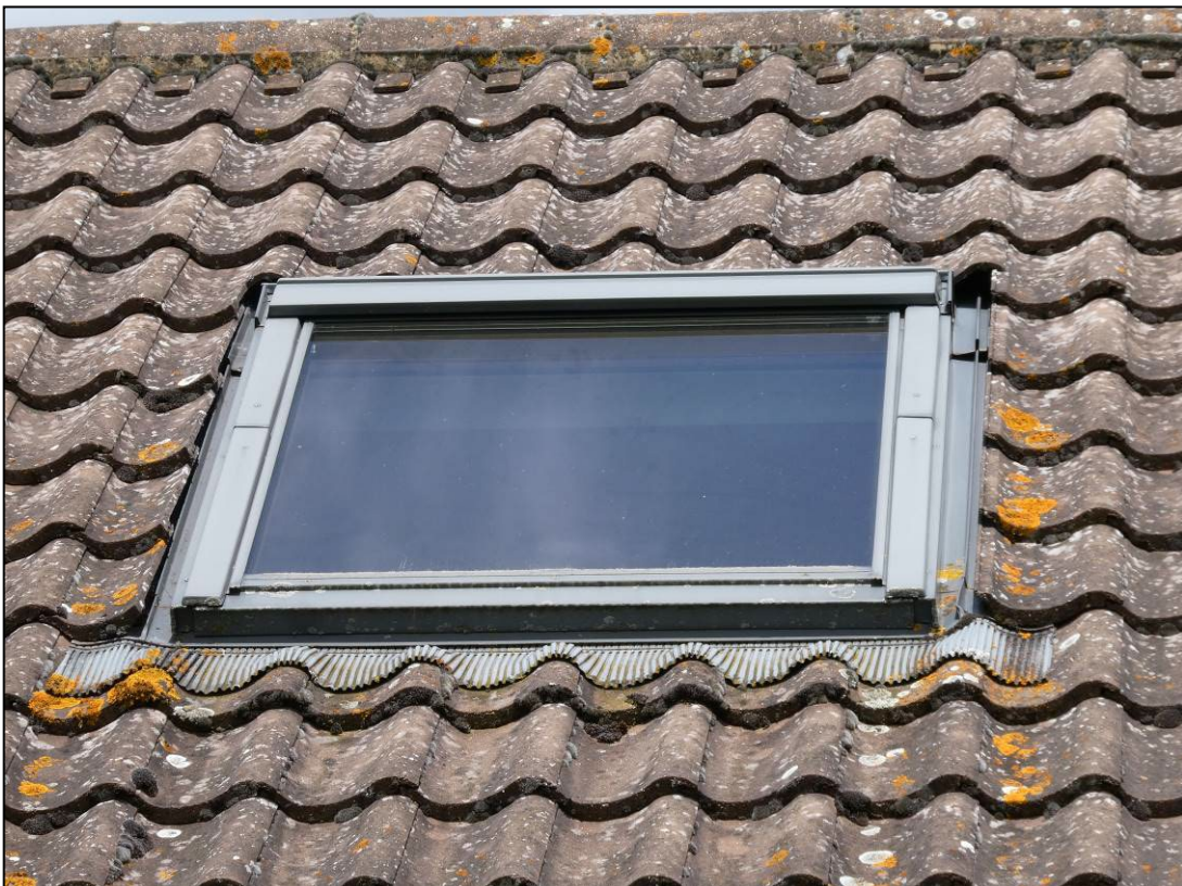
Figure 12. Velux window on garage roof. West Greylake, Part Lane, Riseley. 06.05.24
