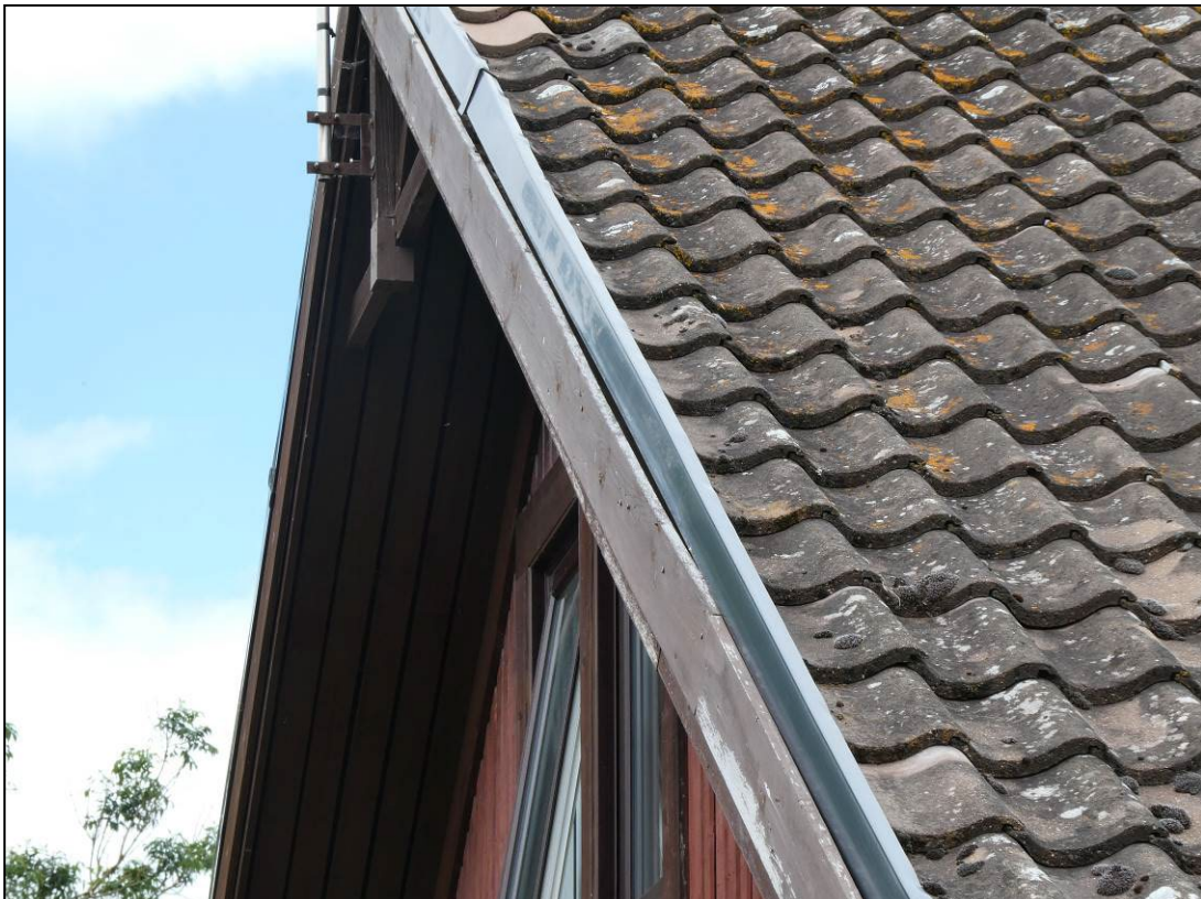
Figure 8. Gaps along the verges. West Greylake, Part Lane, Riseley. 06.05.24
