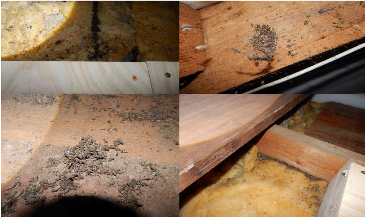
Image 11 – Approx 2000+ bat droppings observed across the floor areas and blockworks to the East gable elevation confirming roosting activity from bats within
