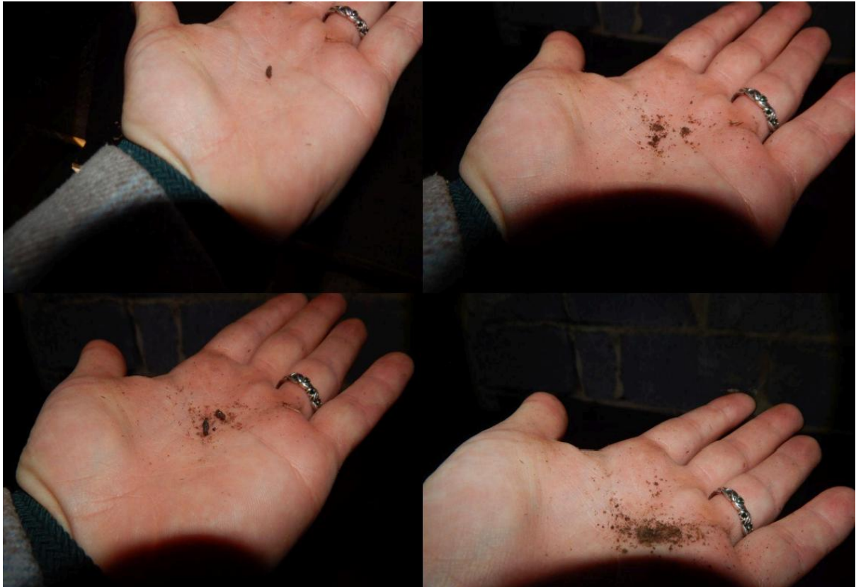
Image 13 – Bat droppings from within the main upper roof void spaces as per images 11 & 12
