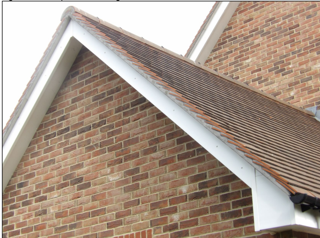
Figure 6. Example sealed verge. 4 Dearlove Place, Shinfield. 30.07.25
