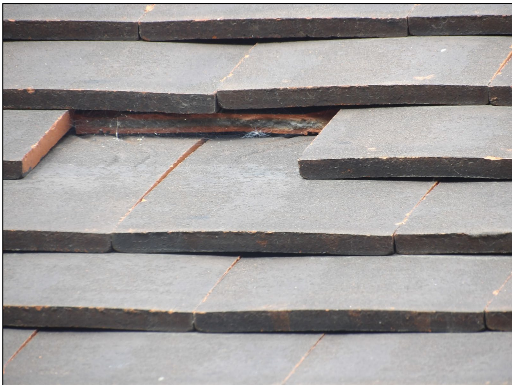
Figure 10. Example broken roof tile on garage with stub in place. 4 Dearlove Place, Shinfield. 30.07.25
