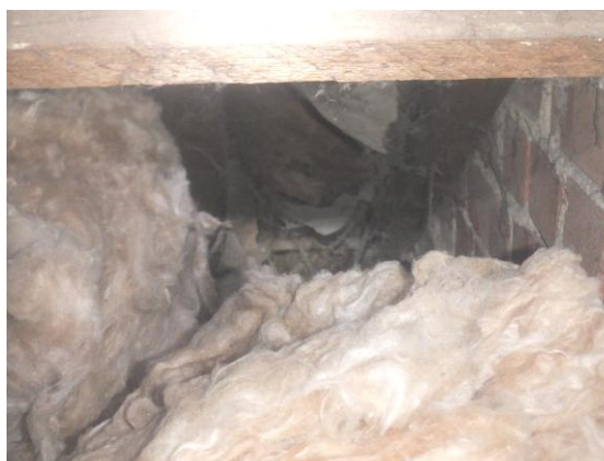
Photograph 12. Bird nesting material within the southwestern eaves.
