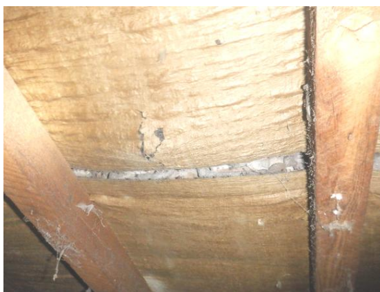
Photograph 9. Torn sections of paper-back felt with roof tiles visible.
