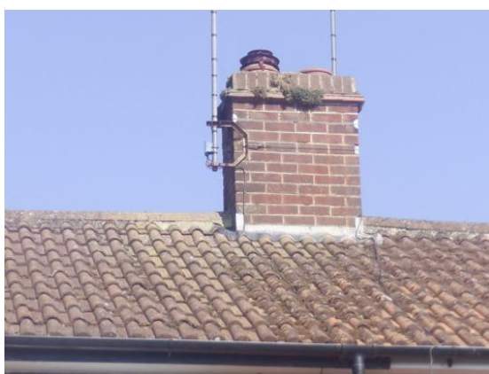
Photograph 5. Lead flashing flat around the base of the chimney (rear elevation).
