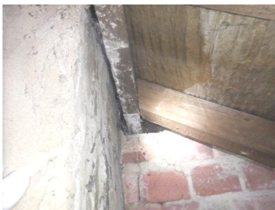
Photograph 11. Gap within northeastern party wall and between rendered chimney and timber.
