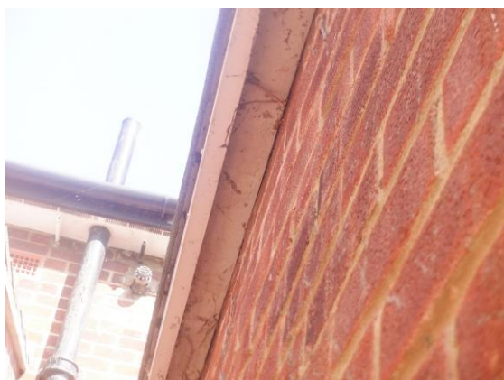
Photograph 7. uPVC soffit tight to brickwork of single-storey extension (western elevation).
