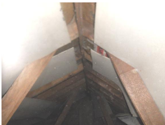
Photograph 8. Void showing roof of cut & pitch construction.
