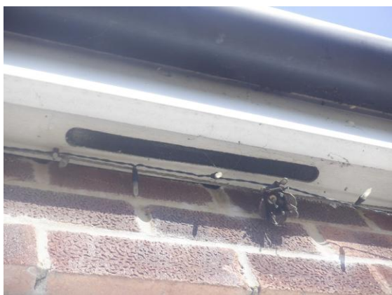
Photograph 6. Vented uPVC soffit sealed to brickwork (rear elevation).
