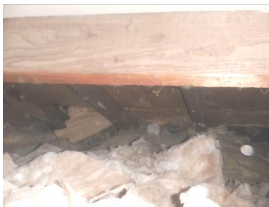
Photograph 10. Fibreglass insulation blocking eaves
