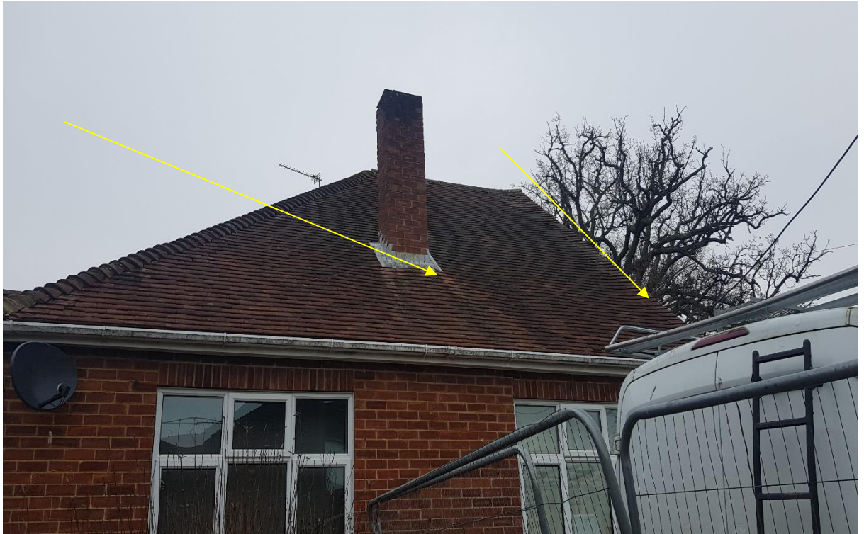
Figure 3: Showing the area the bat emerged on the southern elevation of the property
