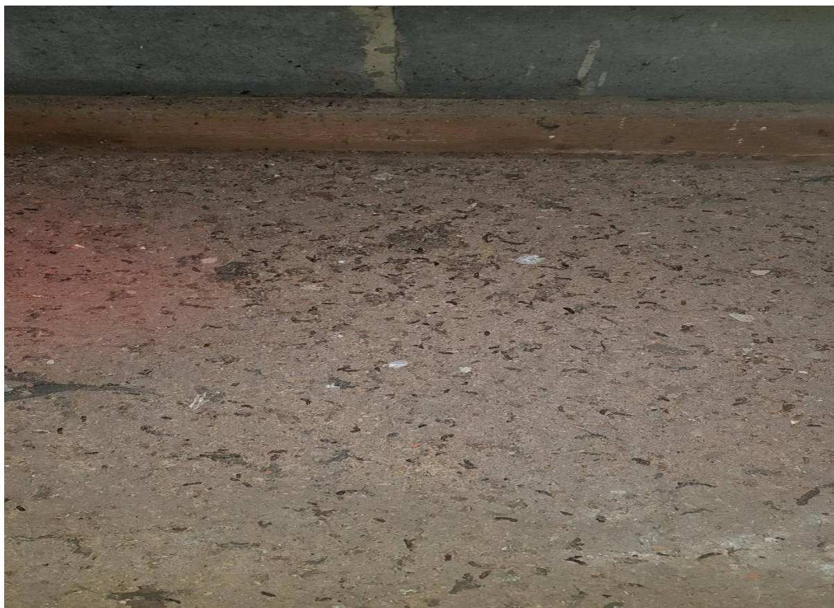
Picture 4: Showing bat droppings in the roof near the front gable wall
