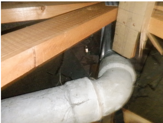
Photograph 13. Large tear in felt around pipe with interlocking roof tiles visible.
