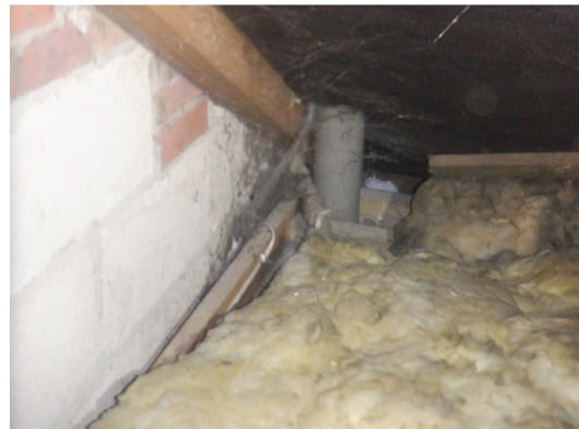
Photograph 14. Large tear in felt around pipe.
