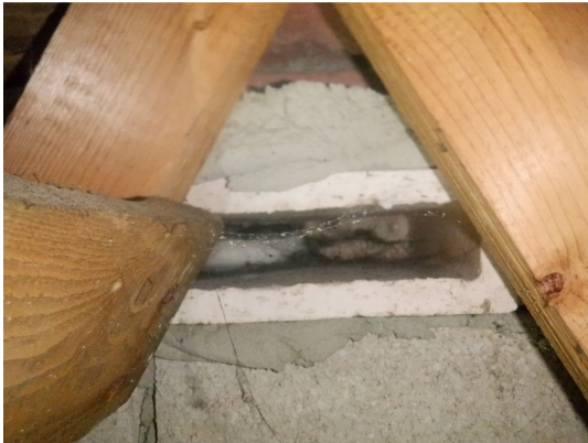
Photograph 17. Vent bricks heavily cobwebbed at apex of gables.
