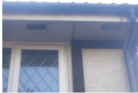
Photograph 8. Asbestos soffit sealed to the house (rear elevation).
