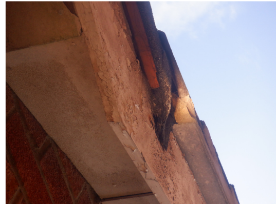
Photograph 6. Superficial crevice within section of crumbling verge mortar (west elevation).
