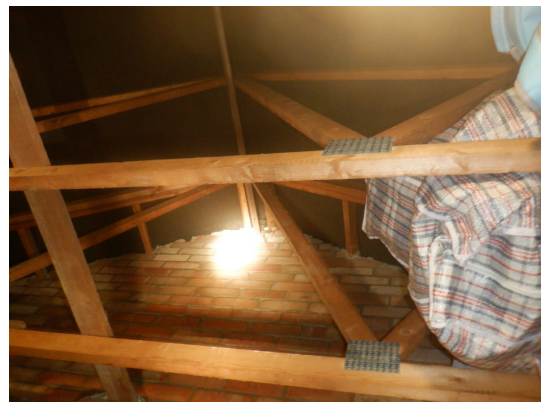
Photograph 19. Gaps along edges of the brickwork gable (garage).
