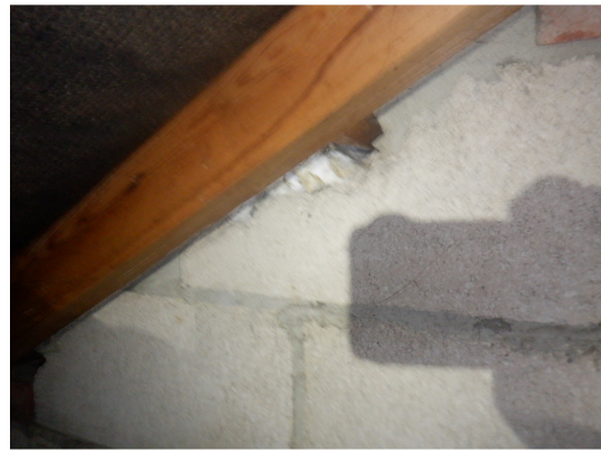
Photograph 16. Gaps at edges of the gables filled with expanding foam.
