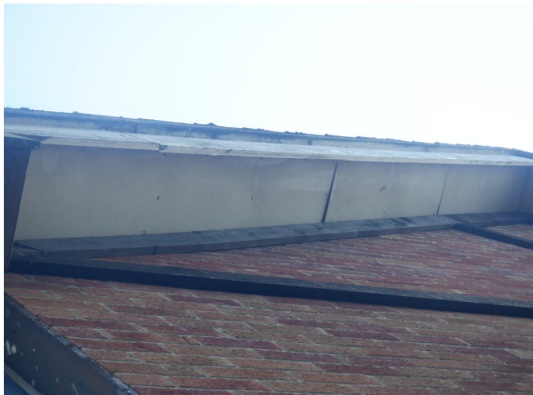
Photograph 10. Mock Tudor timbers sealed to gable (west elevation).
