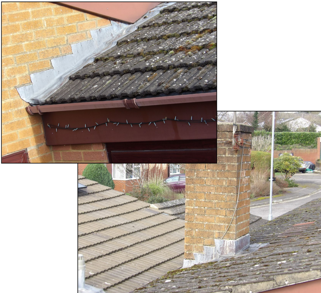
Figure 6. Lead flashing around the chimney and subservient roof section. 79 Wessex Gardens, Twyford. 14.01.25
