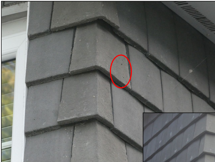
Figure 9. Example gaps in hanging tiles on dormer windows and bat droppings. Lancambria, Basingstoke Road, Swallowfield. 05.08.24
