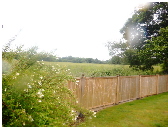
Photograph 4. Slight gaps at the base of the rear timber panel fence.
