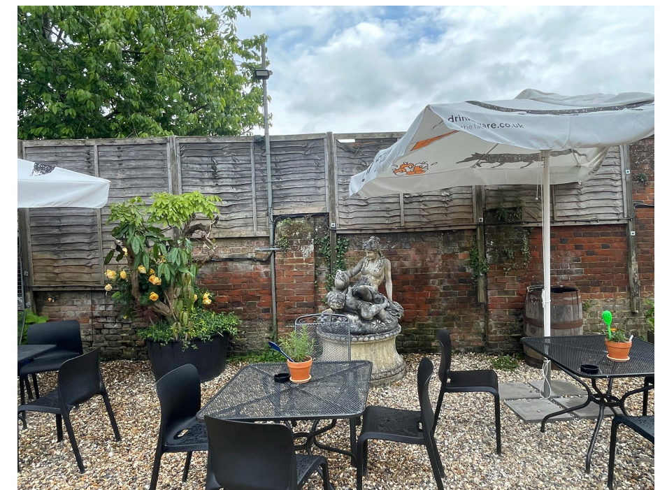
Fig. 30, Garden Wall as seen from the pubs' beer garden and the car park.
