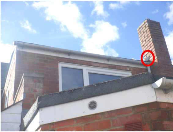
Photograph 6. Lifted bitumen felt at the base of the chimney (rear elevation).
