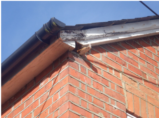
Photograph 9. Gap between timber fascia and verge tiles (southeastern elevation).
