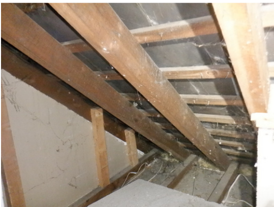
Photograph 14. Gaps situated between insulation boarding and slate roof tiles (northeast eave space).
