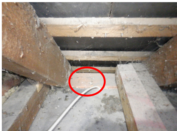
Photograph 16. Bird droppings (southwest eave space).
