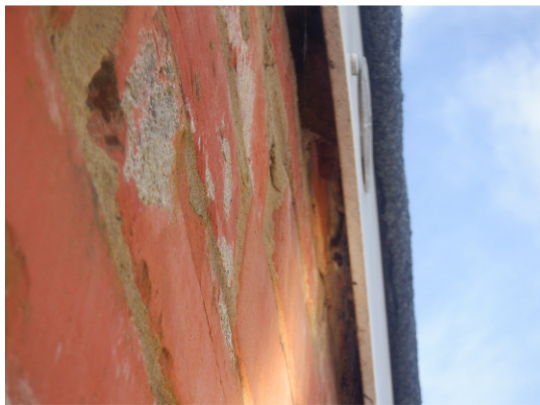
Photograph 10. Gap behind uPVC fascia (rear elevation).
