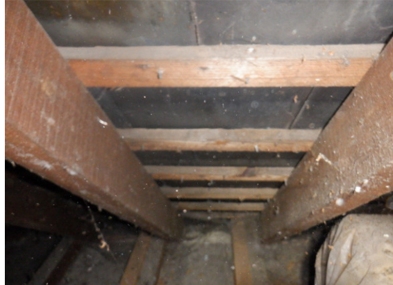
Photograph 12. Unlined roof (Southwest eaves space).
