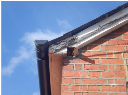
Photograph 8. Damaged section of the timber soffit with direct internal access (southeastern elevation).
