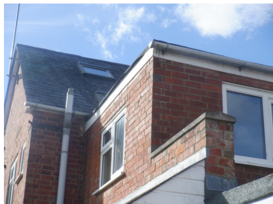
Photograph 4. Hessian-reinforced bitumen felt slightly lifted (southeast elevation).
