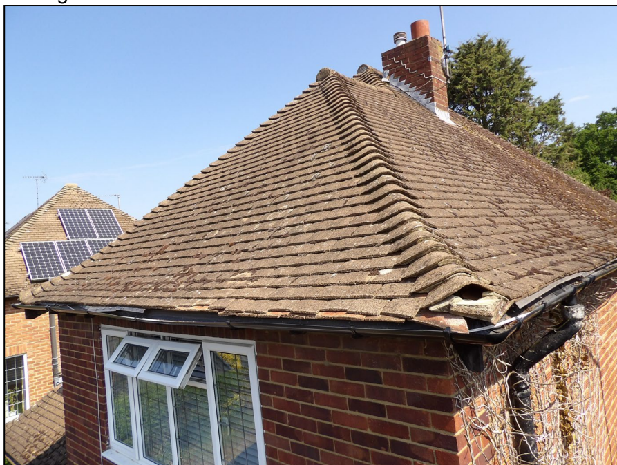
Figure 5. Moved tiles and missing mortar at southeaster roof corner. 26 Priest Avenue, Wokingham. 13.05.25
