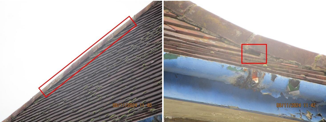
Photo 15 – Gap between wooden fascia and brick wall on the northern elevation of the Church hall, and Photo 16 – Missing verge mortar on the western elevation of the church hall
