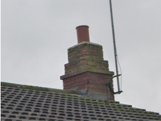
Photograph. 7 Gap of limited extent under slightly raised chimney lead flashing (front elevation).
