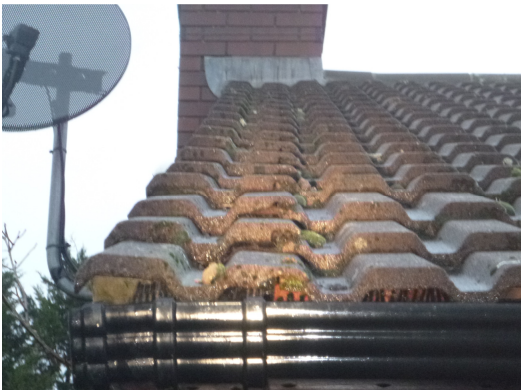
Photograph 3. Lifted interlocking tiles with roof battens visible (rear elevation).
