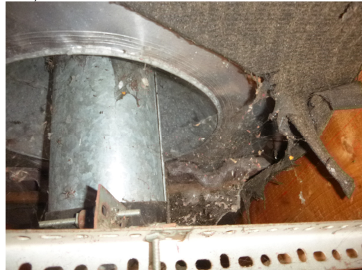
Photograph 11. Tiles visible around pipe (roof void).
