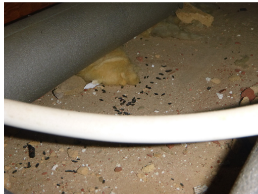
Photograph 13. Rodent droppings (roof void).
