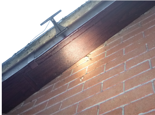
Photograph 6. Superficial gap within crumbling brickwork (northeast elevation).
