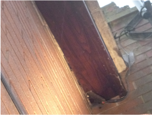
Photograph 5. Heavily cobwebbed gap between soffit and brickwork gable (southwest elevation).
