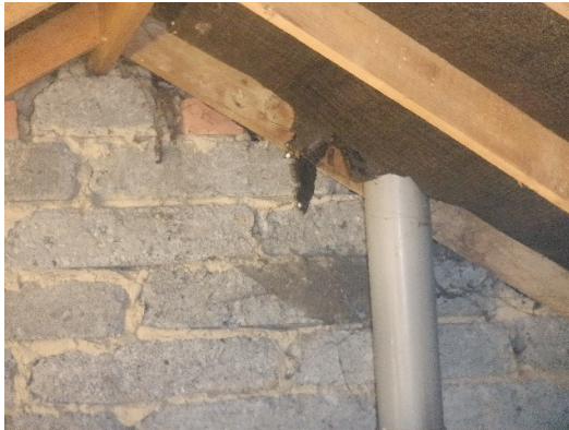
Photograph 19. Small gaps in blockwork, heavily cobwebbed (southern elevation)
