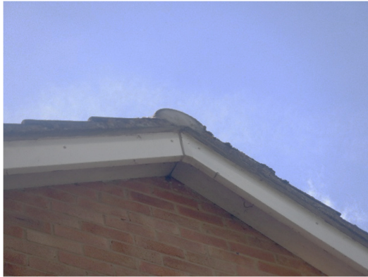
Photograph 5. Minor gap at the apex (rear elevation).
