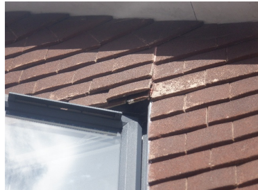
Photograph 8. Lifted hanging tile above the first floor window (front elevation).
