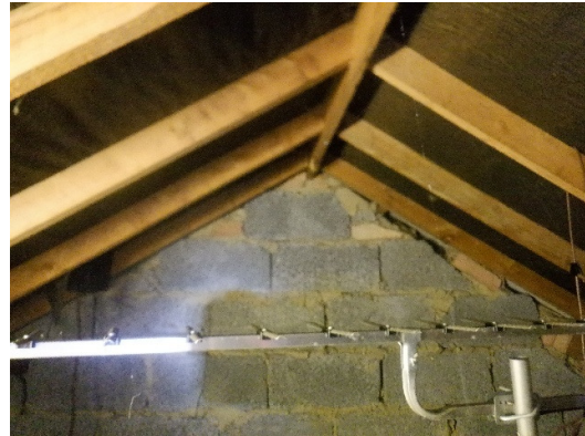
Photograph 20. Small gaps in blockwork (northern elevation)
