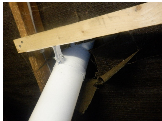
Photograph 17. Torn bitumen felt along the ridge
