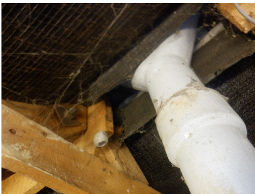
Photograph 16. Loosely fitted bitumen felt along the ridge
