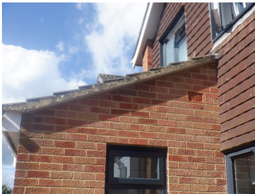
Photograph 13: Porch verge mortar (eastern elevation)
