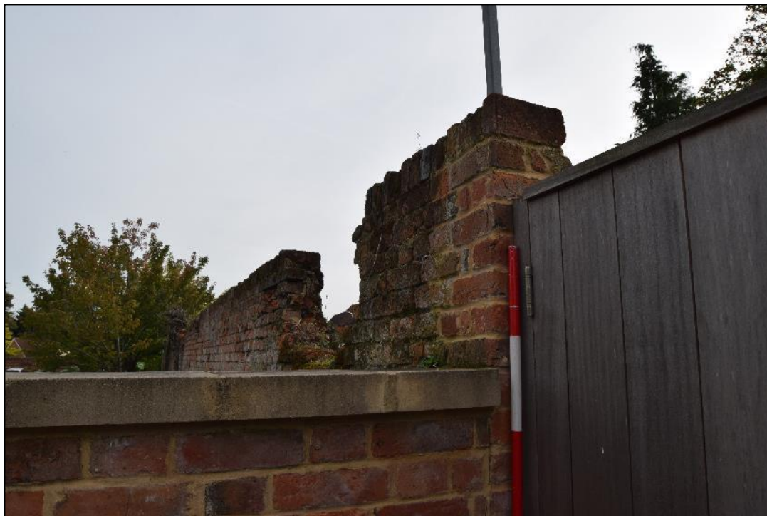
Plate 17: View looking E towards missing upper courses of the NW facing elevation of the wall.
