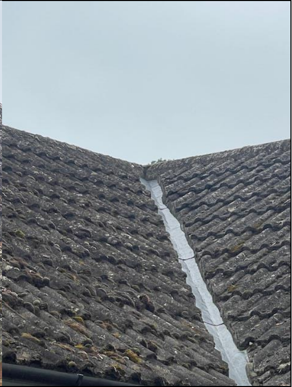
Photograph 12: No gaps around roof tiles.
