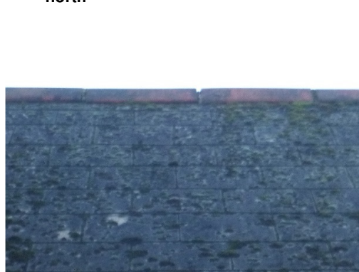
4. Ridge tiles with occasional missing mortar
