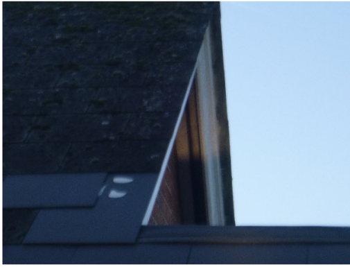
7. Gap behind barge board on extension gable with visible dropping in cobweb
