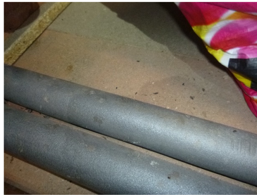
18. Droppings on floor amongst pipe work and stored items
