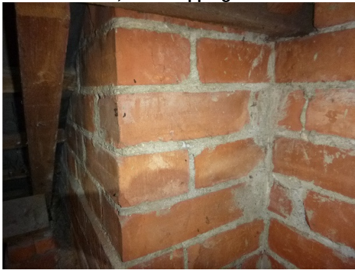
15. Droppings stuck on the chimney wall
