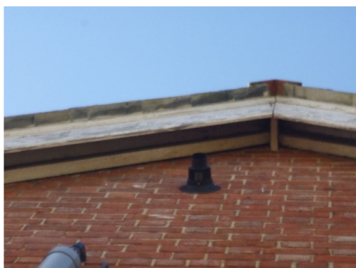
5. Gap behind barge board on eastern gable
