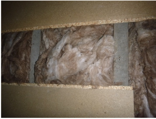
13. Part boarded floor with fibreglass insulation, with droppings
