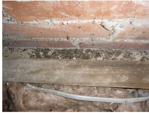
14. Approx 100 dropping at base of western gable end
