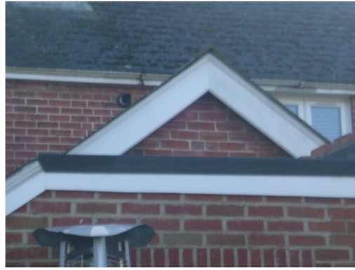
8. Gap in verge mortar apex of extension gable roof
