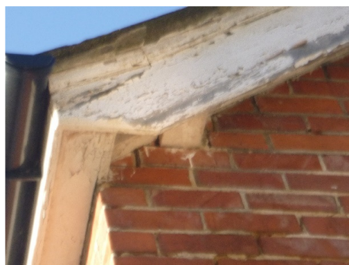
6. Gap around the edges of the brickwork and timber barge boards
