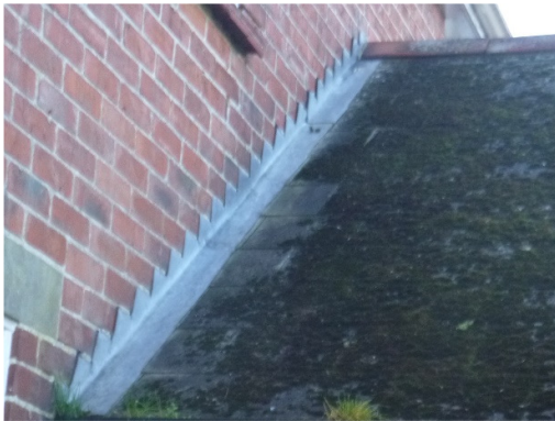
9. Gaps in mortar around lead flashing
