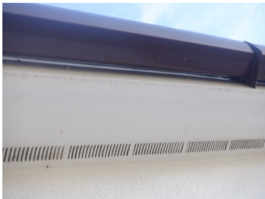
Photograph 6. uPVC soffits tight at the eaves.
