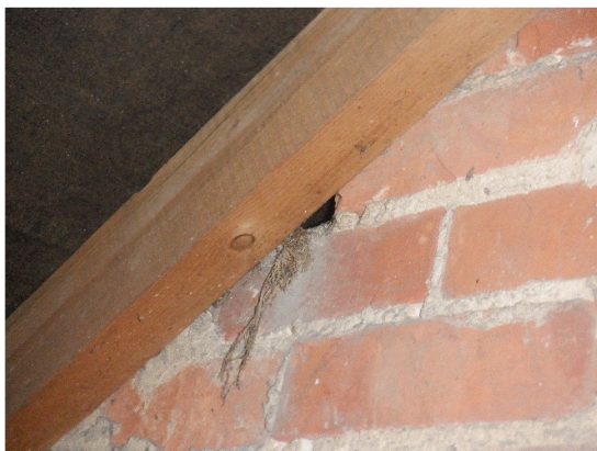
Photograph 15. Slight gaps around brickwork around the gable end.
