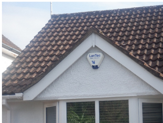
Photograph 7. Fascia tight to the rendered walls at the gable end to the front of the bungalow.
