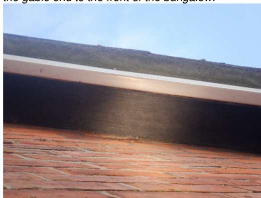
Photograph 9. Superficial gap behind soffit at the eastern side of the bungalow.
