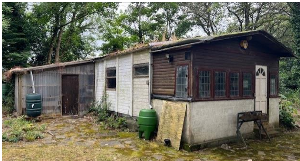
Figure 5: Existing dilapidated building on the site
