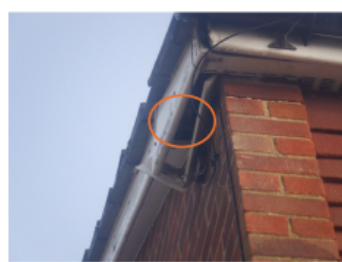
Photograph 16. Broken soffit on northern elevation (TN6).
