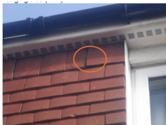
Photograph 13. Gap under top course of hanging tiles (TN4).
