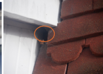
Photograph 14. Gap at hanging tile and uPVC porch join (TN5).
