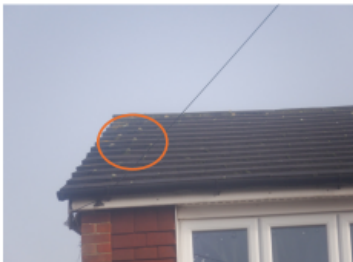
Photograph 3. Lifted tile on front elevation (TN1).
