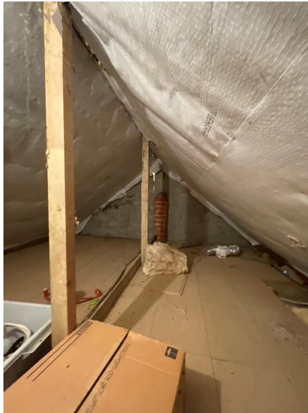
Plate 29: An image showing bat droppings in the interior roof
