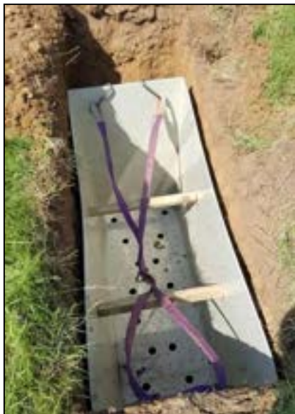
SA-03 with soakaway crate
