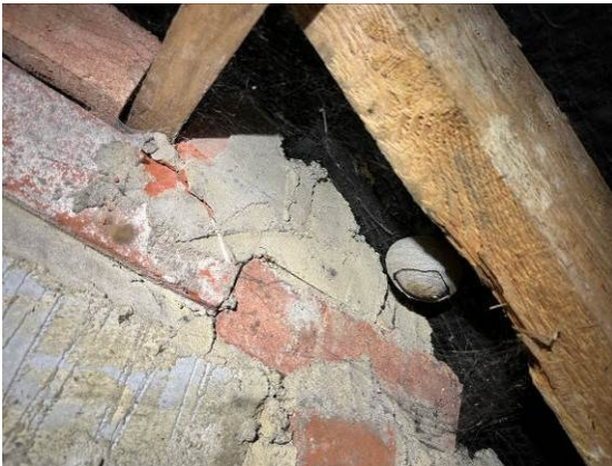
Photograph 15. Gaps over blockwork gable (roof void).
