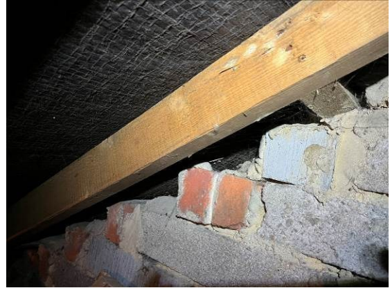
Photograph 14. Gaps over blockwork gable (roof void).
