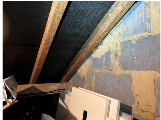
Photograph 16. Gaps over blockwork gable (roof void).
