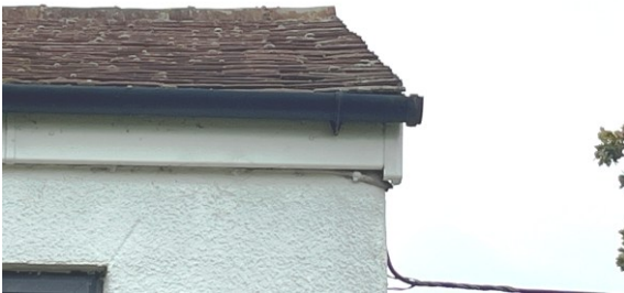
Photograph 9. Occasional gaps beneath verge tiles (eastern elevation).
