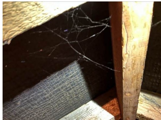
Photograph 12. Cobwebbed ridge and intact bitumen felt (roof void).
