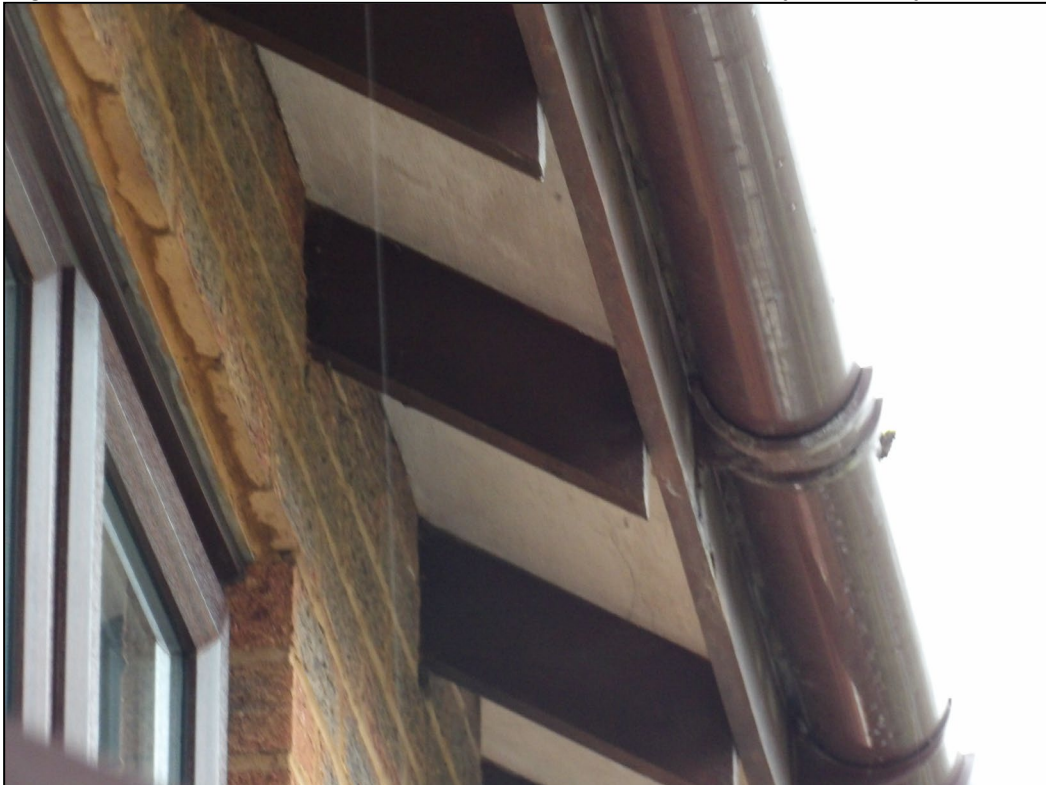
Figure 6. Example sealed eaves and fascias. 22 Beaver Way, Woodley. 17.12.24
