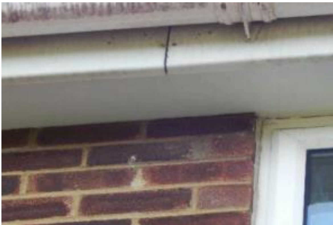
Image 7 – Close view of the rear eaves coverings to demonstrate condition throughout
