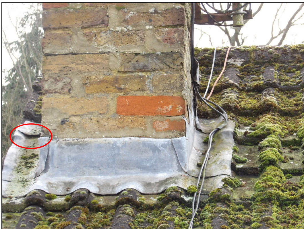
Figure 6. Lifted lead flashing around chimney stack. 216b Nine Mile Ride, Wokingham. 21.01.25
