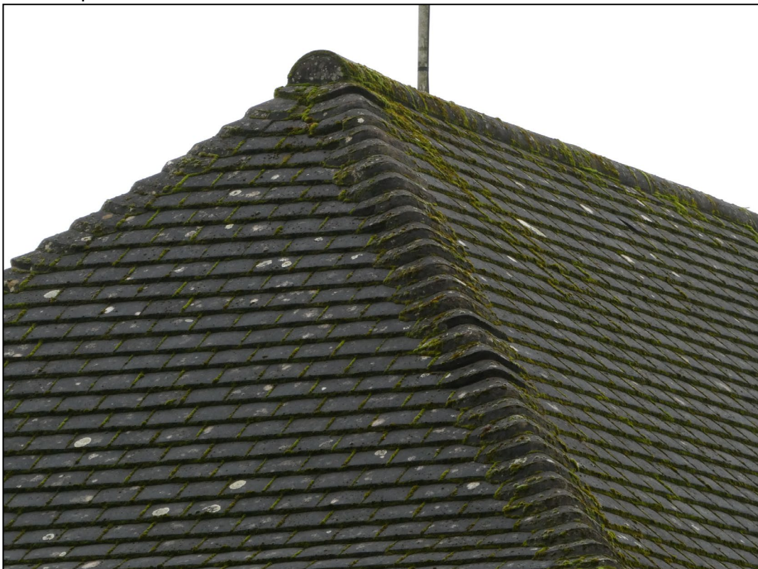
Figure 5. Example of sealed bonnet tiles. Brook House, Hollybush Ride, Finchampstead. 05.12.23
