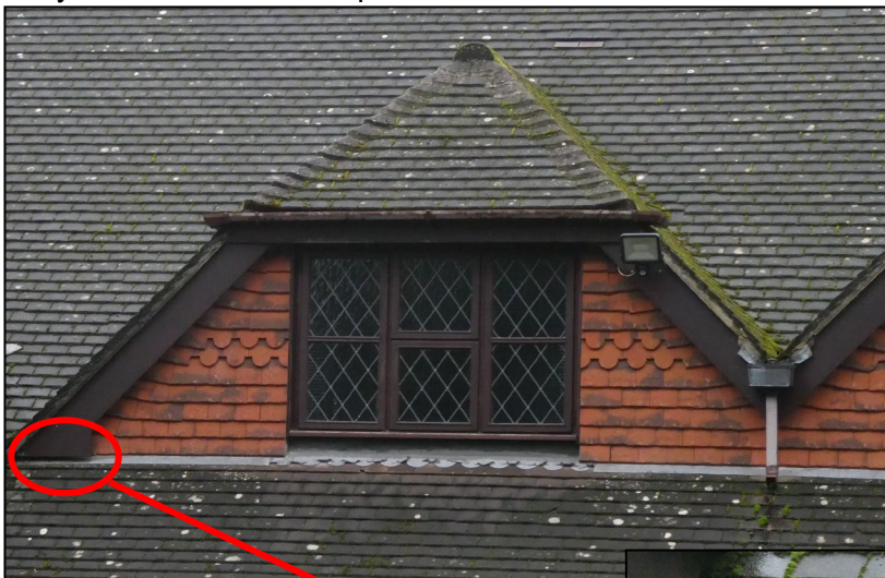
Figure 9. Example dormer windows and gaps on front elevation. Brook House, Hollybush Ride, Finchampstead. 05.12.23
