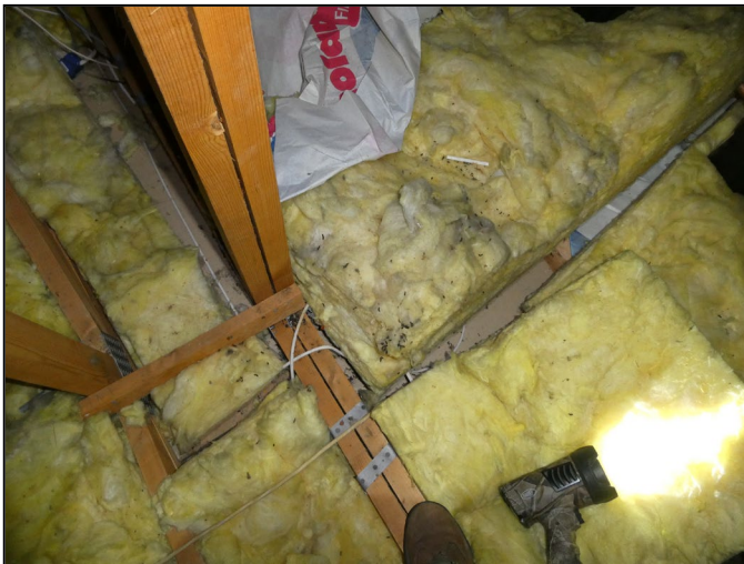
Figure 12. Example of bat droppings. Brook House, Hollybush Ride, Finchampstead. 05.12.23
