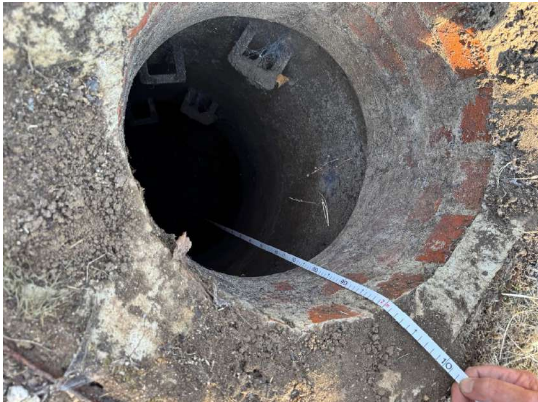
Storm drain with metre measure. Depth 2 metres plus thick mud at the bottom, total 2.5 metres= 8 feet deep.
