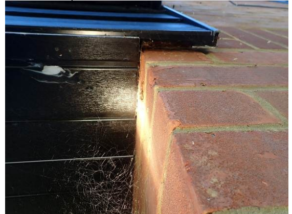
Photograph 6. A narrow gap behind fibre boards at junction with wall.
