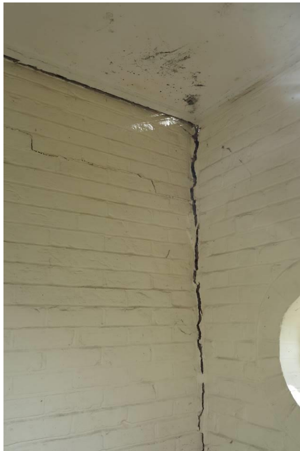
Plate 22. The porch is coming away from the western elevation of the house
