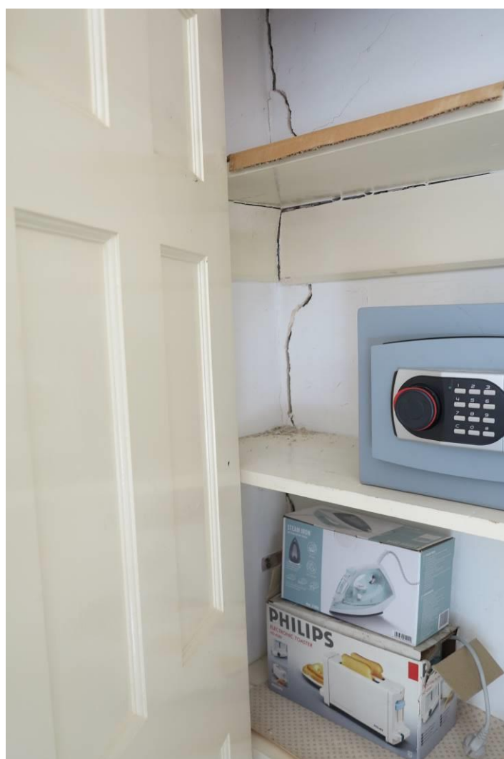
Plate 20. Cracks are evident to external walls throughout the building
