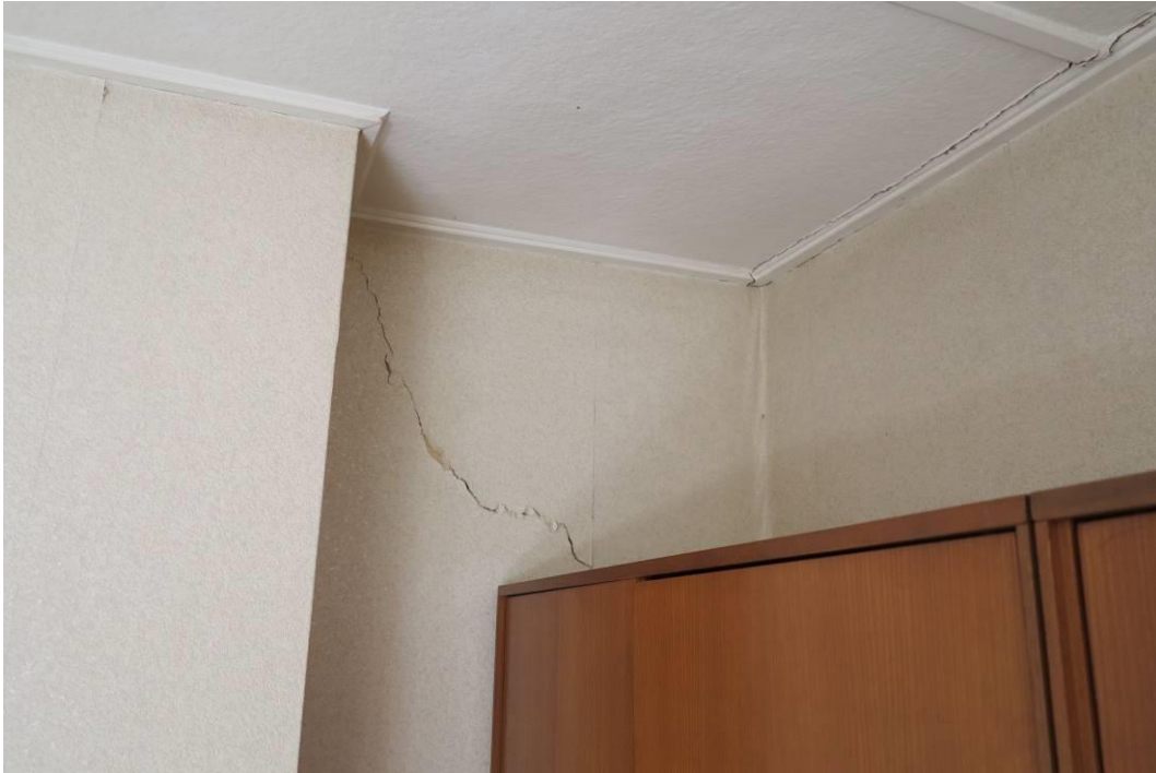
Plate 21. Cracks are evident to external walls throughout the building
