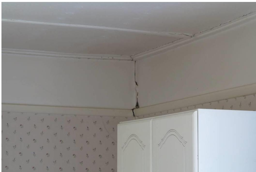
Plate 19. Cracks are evident to external walls throughout the building
