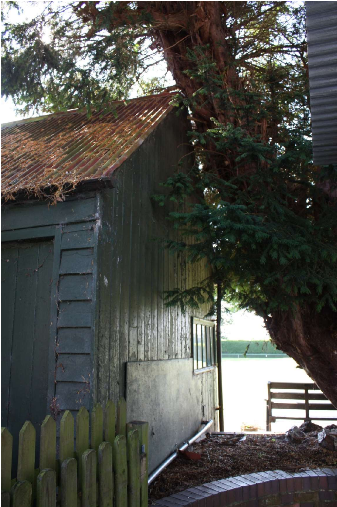
5. West gable from Pub grounds shows disused door.
